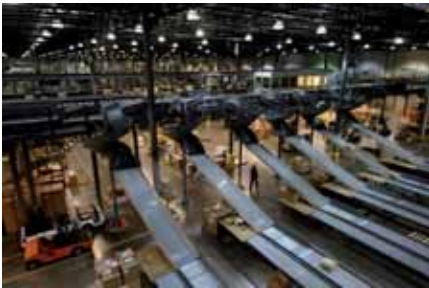
Complex conveyor systems have potential for significant energy savings
