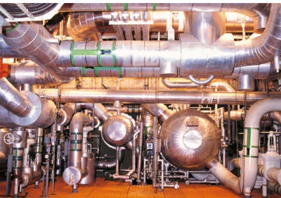
Optimum energy efficiency, e.g. in complex pumping applications
